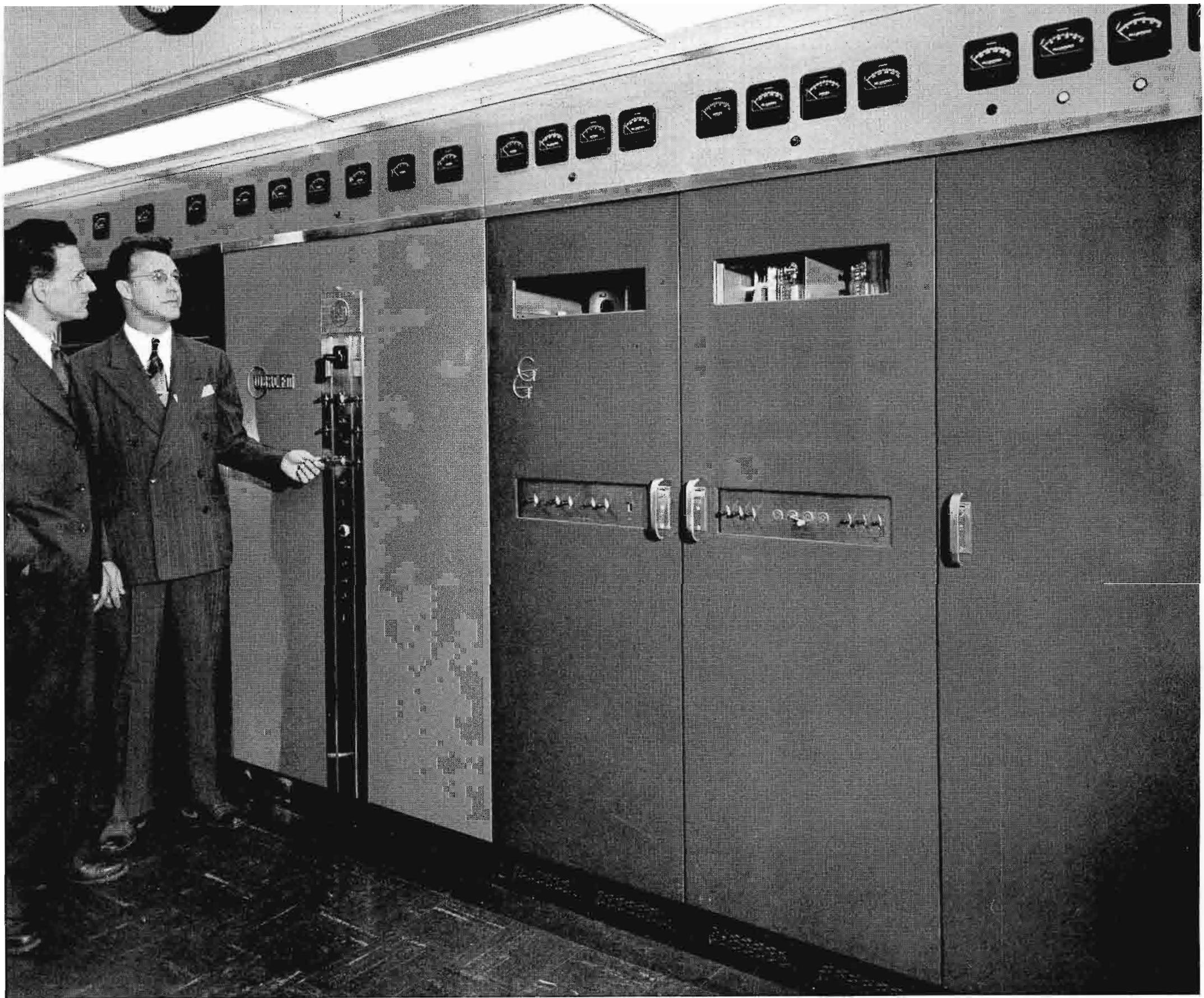
FIG. 2 (above). WBRC-FM's 50 KW transmitter, RCA type BTF-50A, presents a streamlined appearance, with all essential controls front-panel mounted and easy to reach. In this view G. P. Hamann, author, is at the controls while C. J. Starner, RCA engineer, looks on.
