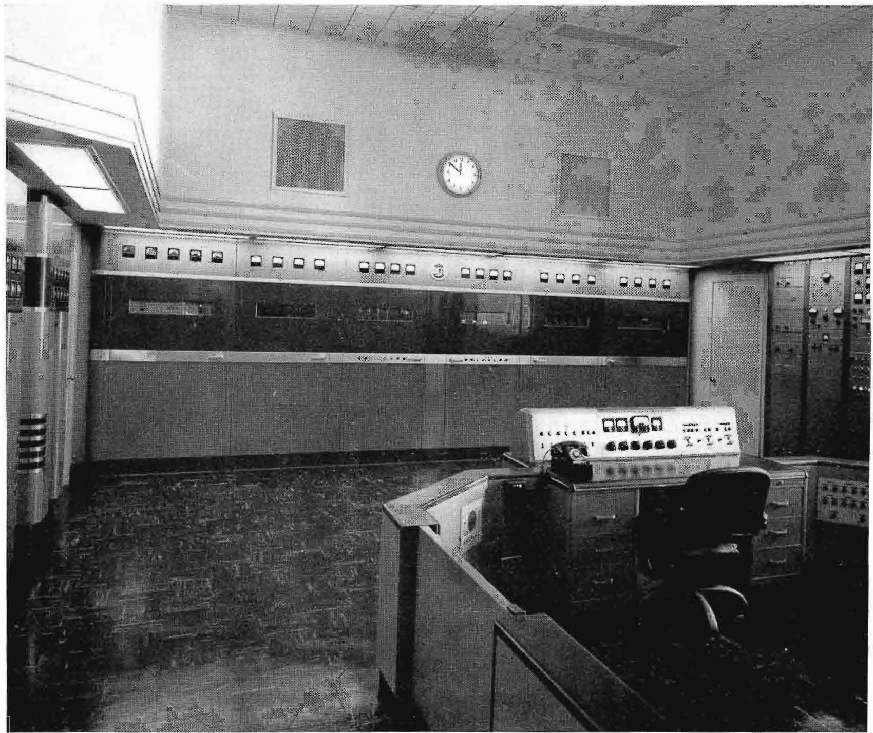
FIG. 2. The station is as neat looking inside as outside. Shown at right is the transmitter room which contains a 10 KW RCA Type BTA-10F Transmitter, a 1 KW BTA-1L Standby Transmitter, the speech input equipment, and the operator's control console.
