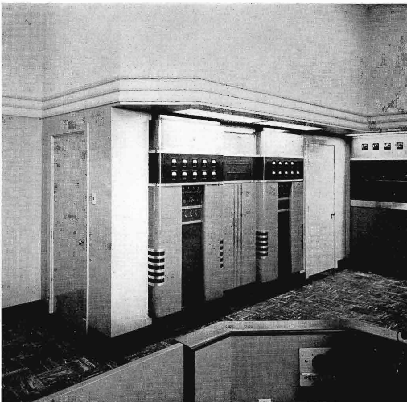
FIG. 4. Above is the 1 KW RCA Type BTA-1L emergency standby transmitter. The unit is mounted flush in a drop wall. Doors on either side permit easy access to the rear of the transmitter for servicing.
